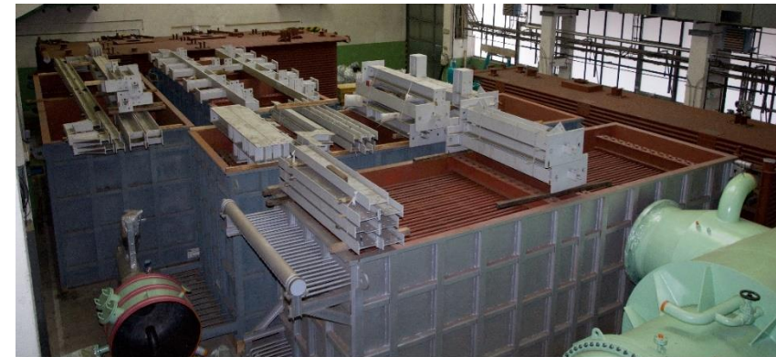
ECO modules 1-6 + steel structure
